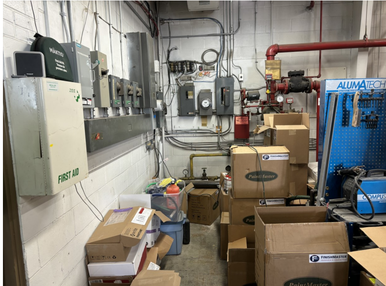
Sprinkler & Hydro Area
